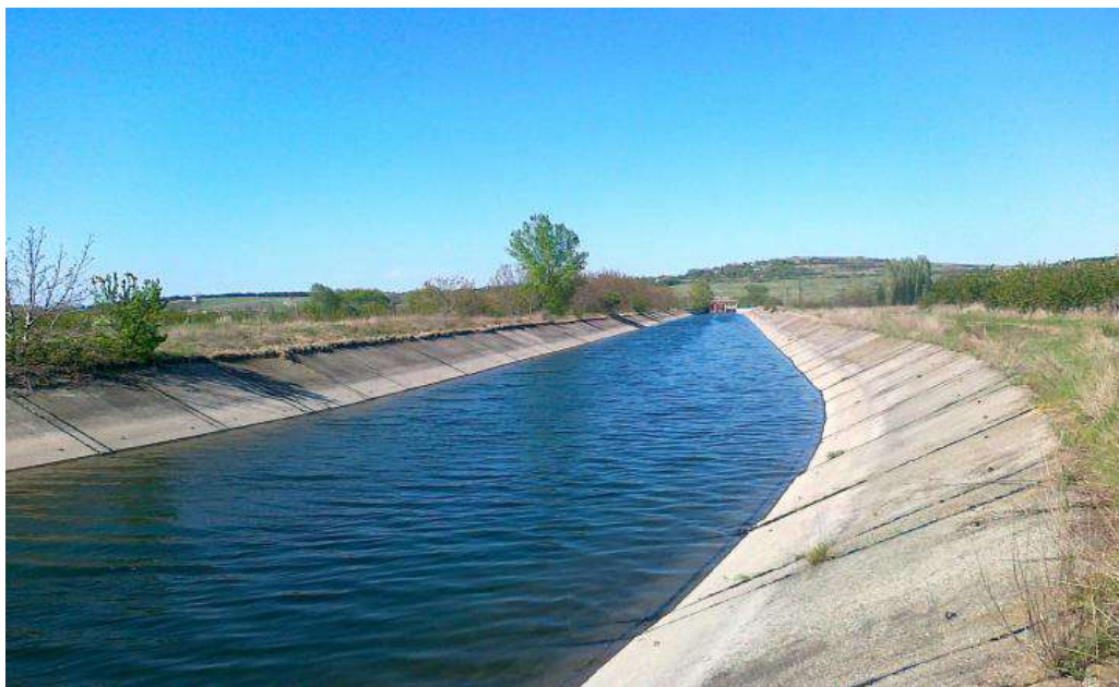
Figure 51 - Chanel of Irrigation systems EAD
