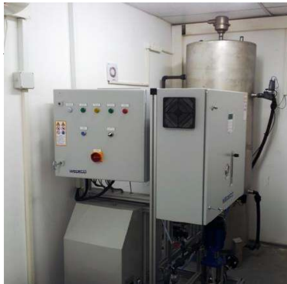
Figure 3 - ozonator at the Shafdan WWTP R&D center
