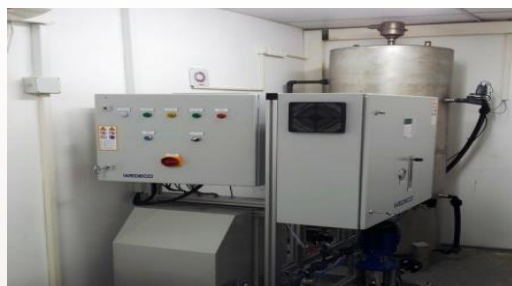
Figure 3 - ozonator at the Shafdan WWTP R&D center
