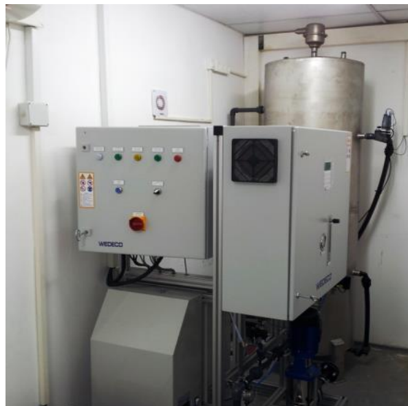
Figure 3 - ozonator at the Shafdan WWTP R&D center
