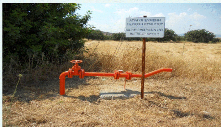
Picture 2 – A pipe carrying reclaimed water to agricultural fields for irrigation in Nicosia, Cyprus. Pipes carrying reclaimed water are painted red to be distinguished from other water pipes.
